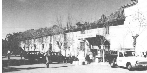
Figure 36. Poor Plaster applied on Walls (Altınsapan, 1999: Figure 6)
