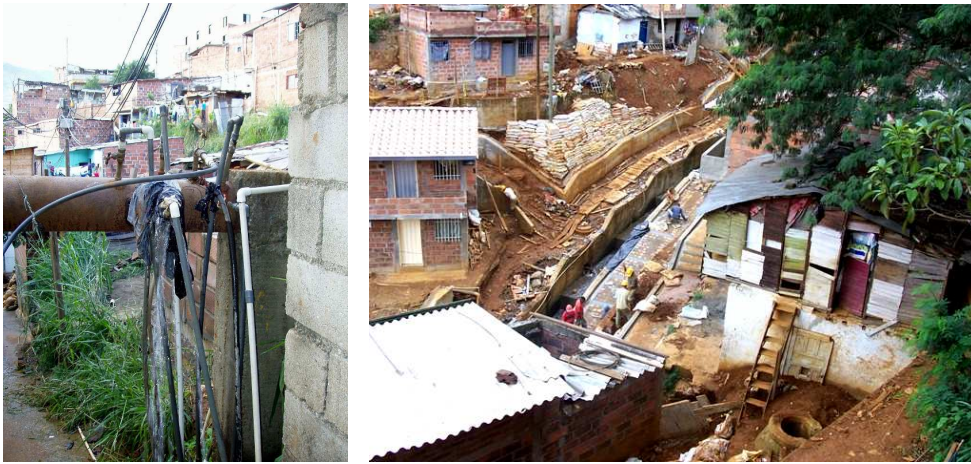
Fig. 2. Illegal water installations. Fig. 3. Opening space for public services and common areas.
